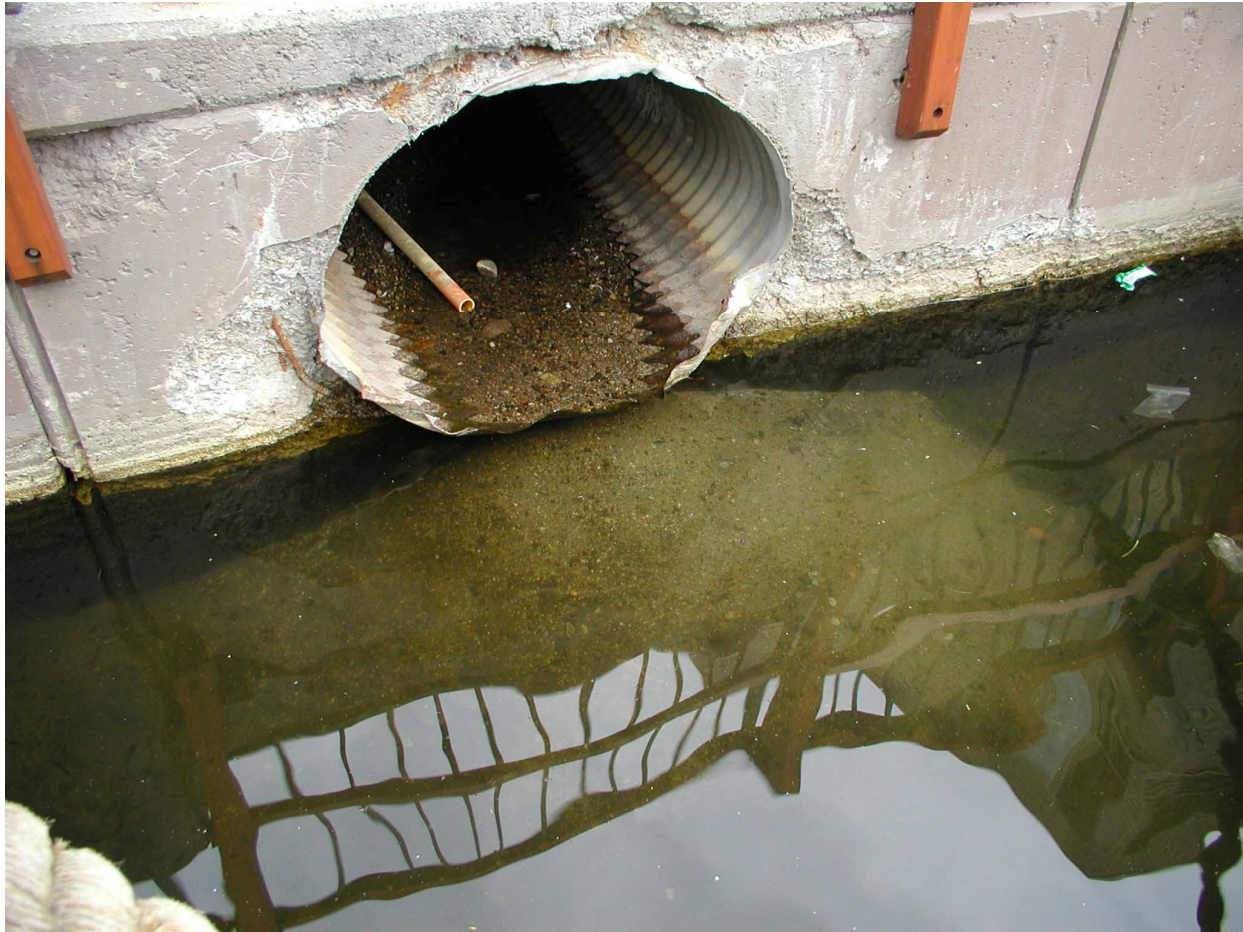
Figure 5. Bedload sediment accumulation in sewerage and near inlet to pond (Snowmass, CO).
